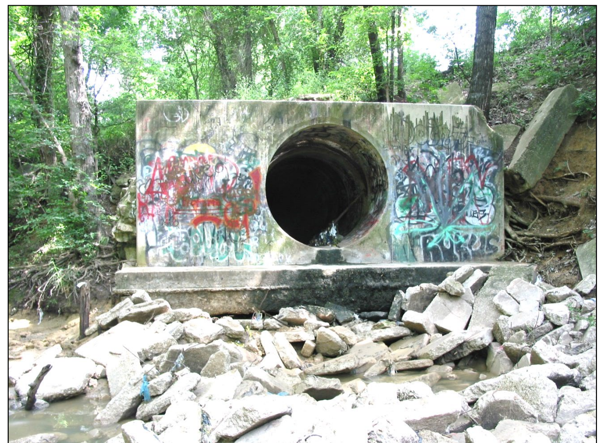
96" RCP Outfall near Christopher Drive (Pipe separated from headwall)
